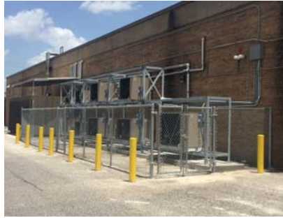
Texas Department of Health and Human Services (HHSC)- Richmond State Facility Refrigeration System design for food services warehouse
