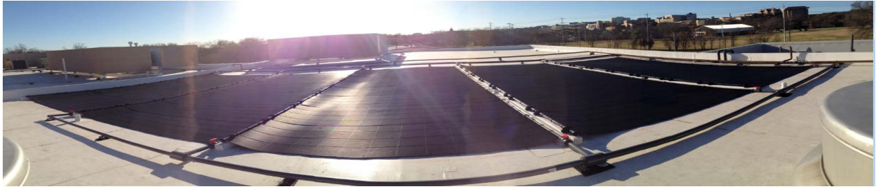
City of San Marcos - Solar Thermal Pool Heating at San Marcos Activity Center. (MEP by TEESI)
