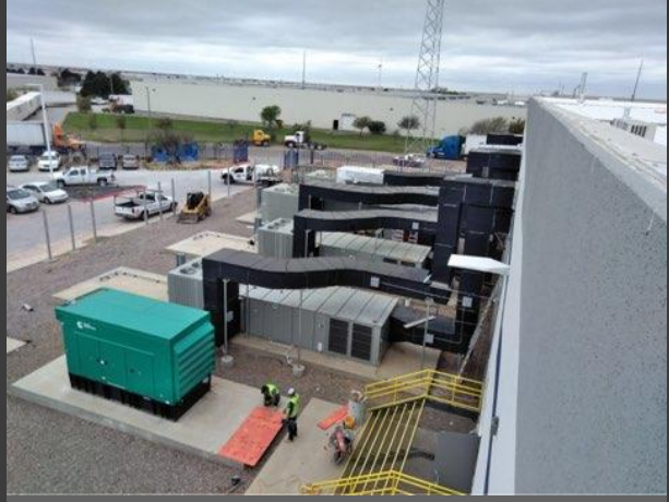
Exterior Mechanical Yard
