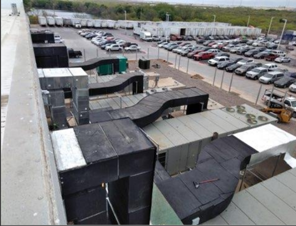
Exterior Mechanical Yard
