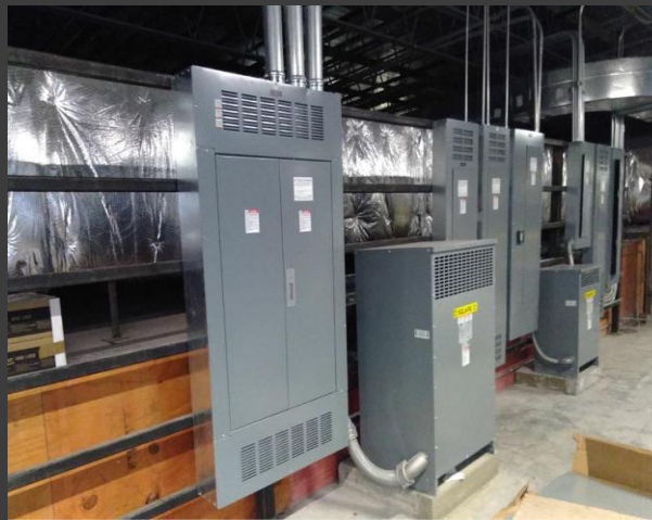
Electrical Distribution Panels
