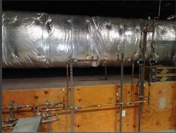
Air Compress System
