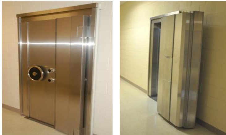
The Level 5 door of the Long-Term Storage Vault (same model used for each vault).
