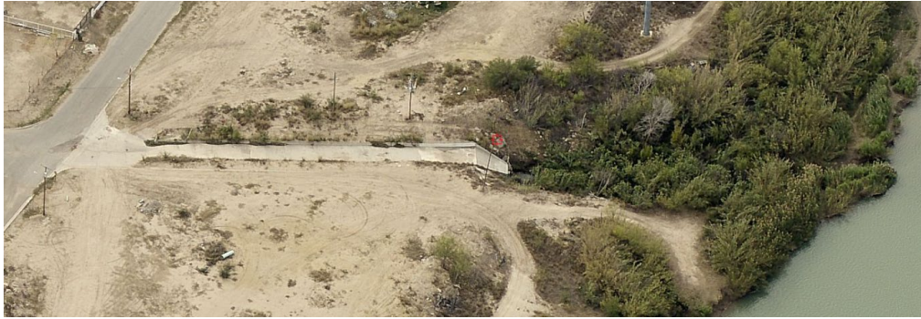
Figure 2—Centeno Lane outfall into Rio Grande showing newly built concrete chute into existing outfall channel with vegetation downstream cleared (ca. January 2013)
