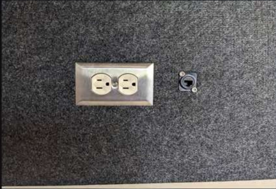
Wall Mounted Power for TV/ Kiosks
