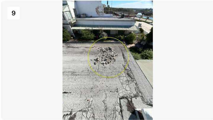
Debris on roof
