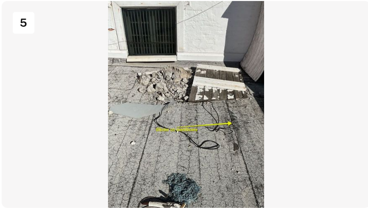
Blister on roof membrane
