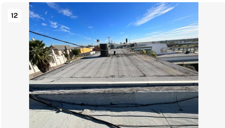
Severe wear & tear on roofing membrane
