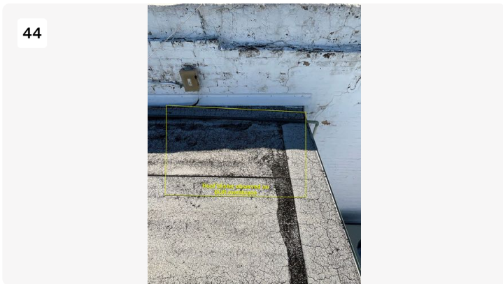
Roof blister observed on BUR membrane
