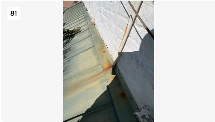
Voids on counter flashing sealant
