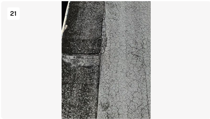
Base flashing coming undone
